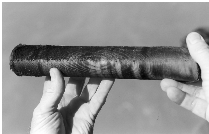
Core samples, such as this one, show that many of the pilings are in good shape, but some have been damaged.
